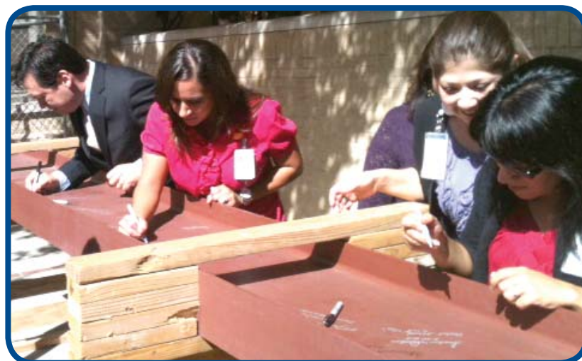
Staff members add their signatures on the last piece of steel for the new building on Robert B. Green Campus.
